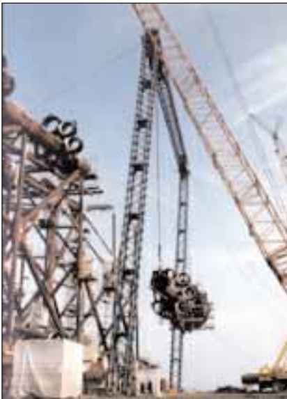
Above: bottle at end of first stage of lift with tower ready for luffing to the vertical.
