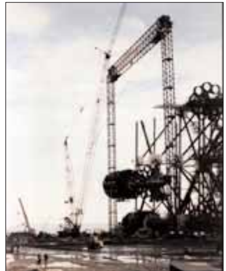
Above: completion of lift with towers luffed in opposite direction for final positioning.
