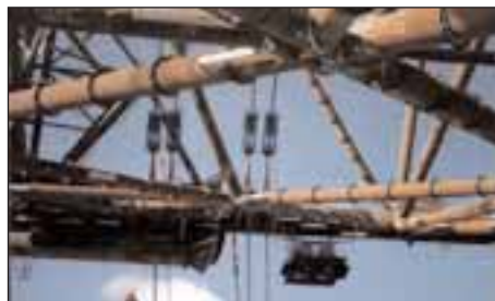
Top: jacks in tension frames sling connected to outer edge of panel.
