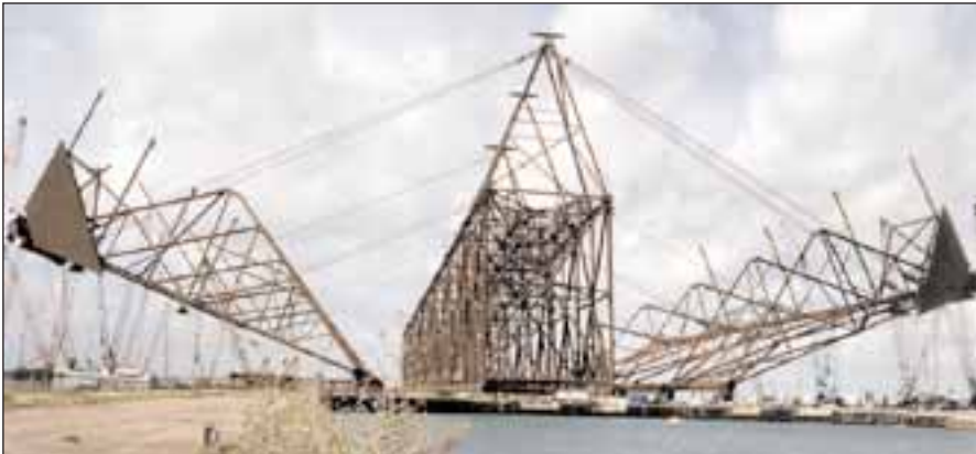
Above: roll-up at 30° just prior to assisted crane release on to jacking system.
